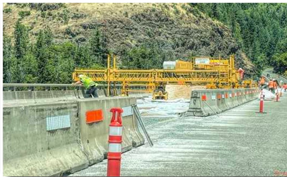
Once you get the green light to cross the bridge over Lost Creek Lake - be prepared to drive very slowly and keep one eye on the narrow lane and the other on the many construction workers. Photo by Christy Solo
